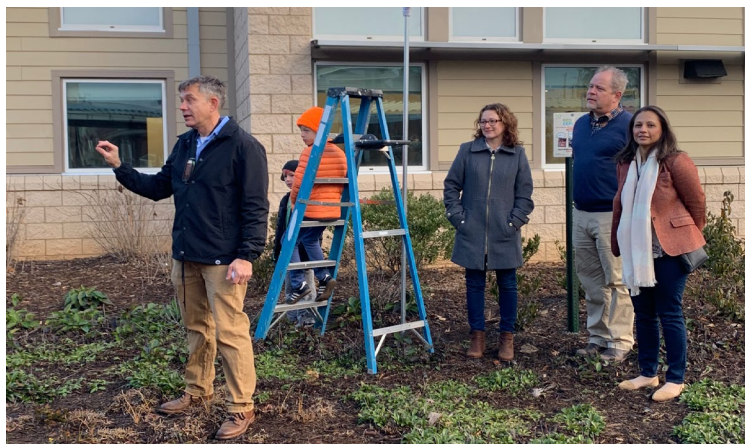
Figure 2. Jenny Disson (right) and Jessica Matthews (third from right) from CISESS join Matt Menne of NCEI (left) at the installation of a weather monitoring station at Isaac Dickson Elementary School in Asheville, North Carolina.
